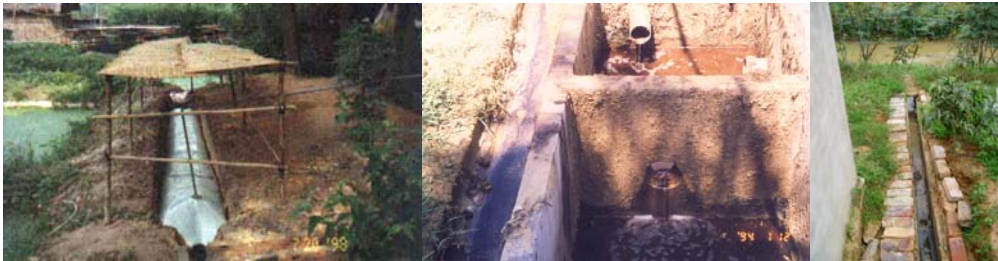
Manure management technologies on Vietnamese farms, left to right; tube biogas digester, sedimentation tanks and channel transport of slurry directly discharged to recipient.
